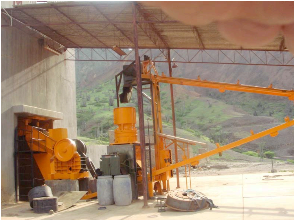
Crushing circuit with a 90% overhaul
