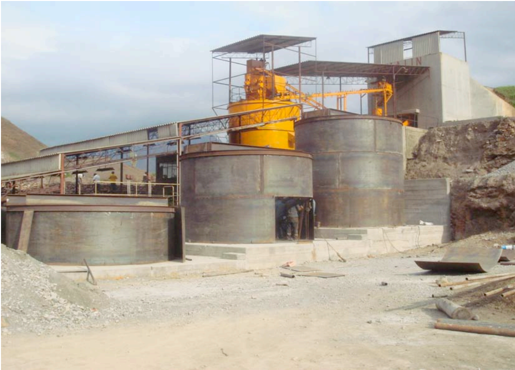
Lateral view of the new leaching tanks
